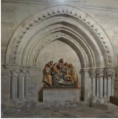
Gothic doorway of the cloister of the collegiate church of Santa María la Mayor
